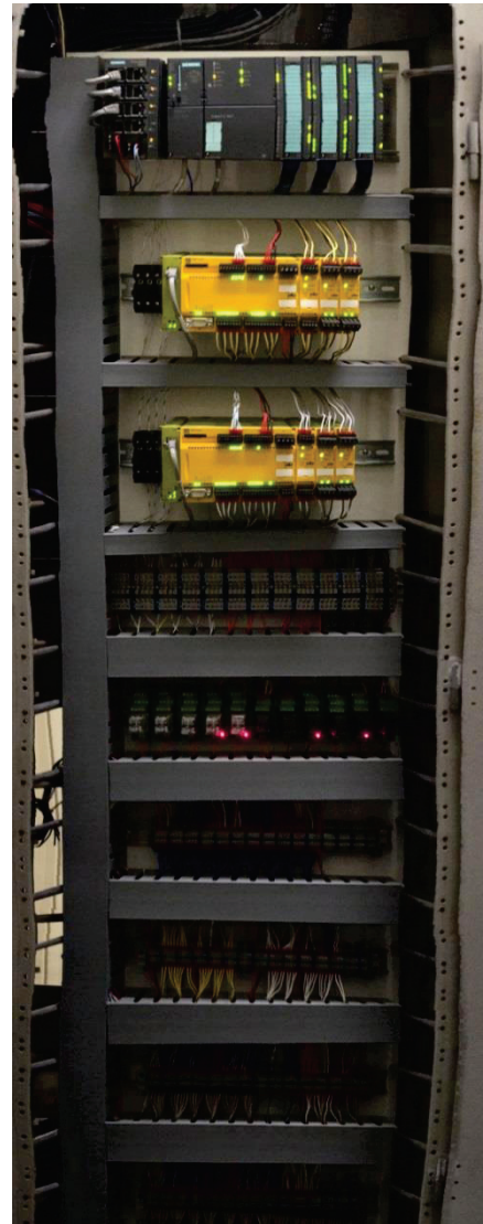
Figure 2: New Installation in repurposed racks.
