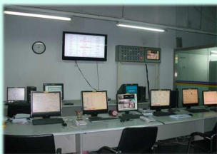
Cryogenic Control Room
