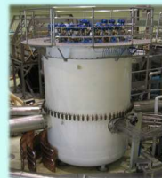
Distribution Valve Box
