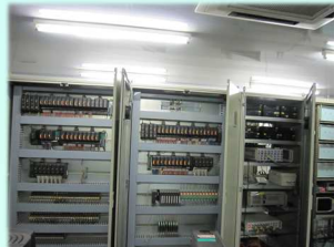
Local Control Cabinet
