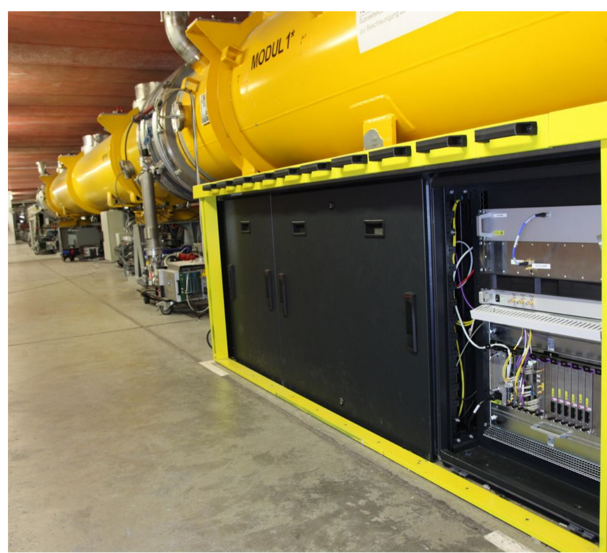
MicroTCA.4 LLRF installation in the FLASH accelerator tunnel
